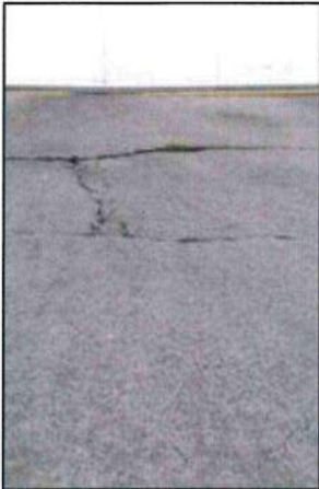
Photo 29 – Fire Station #1 The concrete at the garage is severely cracked and deteriorated. Loss of underlying support is also evident as a result of possible washout or settling.
