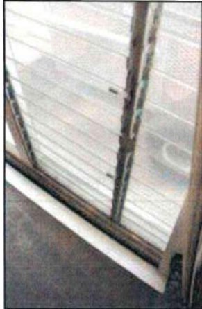
Photo 49 – Fire Station #1 Windows show deteriorated frames. The outdated louver windows allow air and moisture intrusion.
