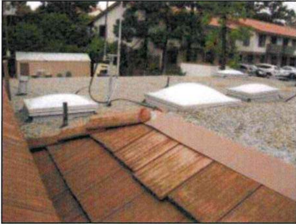
Photo 17- Fire Station #4 The pitched roof is a clay composition tile with metal flashing, skylights, and a portion of the flat roof with gravel overlay.
