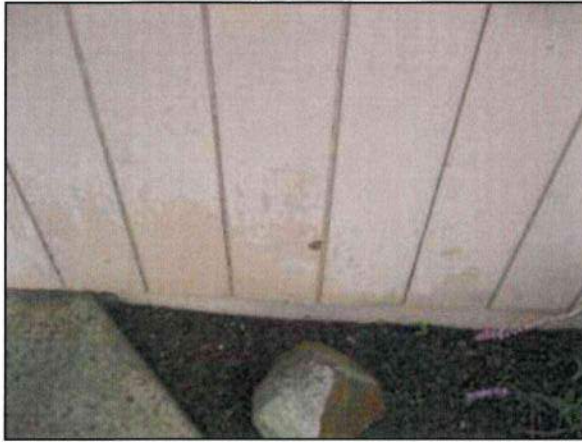
Photo 33 – Fire Station #4 The fire station structure is sheathed in 5/8" T-111 plywood siding.
