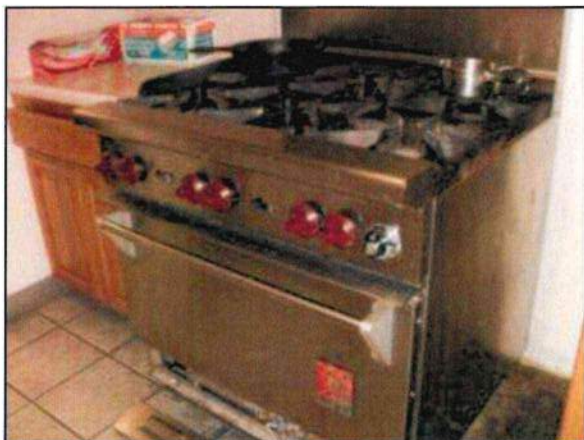
Photo 21 – Fire Station #1 The commercial-grade gas range and oven unit requires a thorough cleaning. The ceramic tile underneath requires repair in order to address sanitation.
