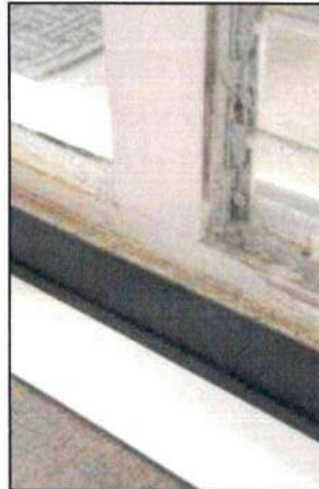
Photo 50 – Fire Station #1 Windows show deteriorated frames. The outdated louver windows allow air and moisture intrusion.
