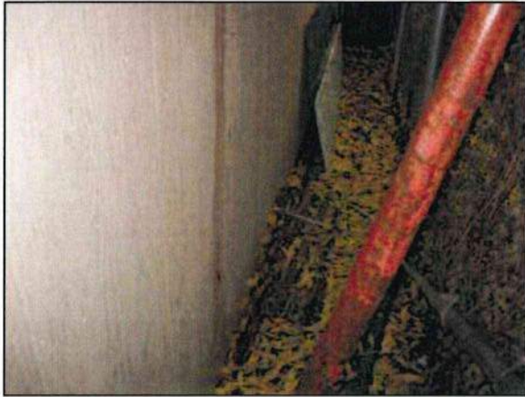
Photo 49– Fire Station #4 The back side of the storage shed is beginning to rot due to the presence of wet debris.
