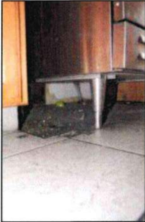
Photo 45 – Fire Station #1 Flooring around the kitchen range is missing and debris has accumulated.
