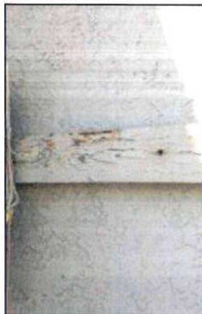
Photo 35 – Fire Station #1 Exterior wood trim exhibits cavitations, heavy rot and peeling of paint, and possible termite damage.
