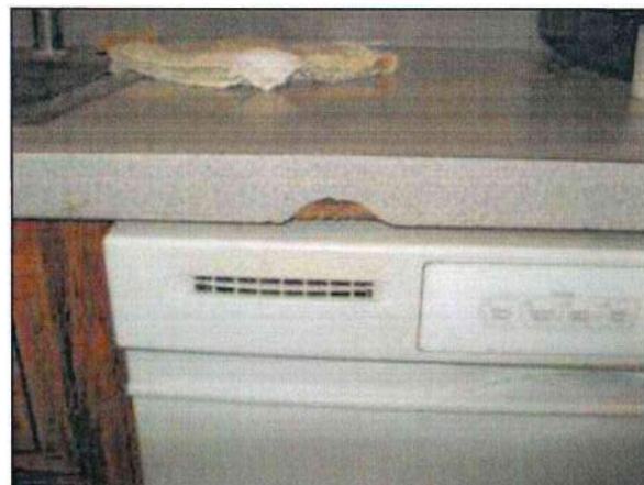
Photo 64 – Fire Station #4 Damage to the Formica countertops is present in the kitchen.
