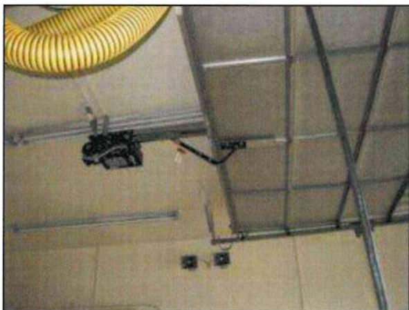
Photo 11 – Fire Station #4 The garage door is powered by an electronic Liftmaster opener.
