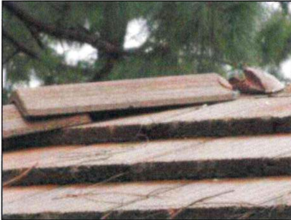
Photo 25– Fire Station #4 Unsecured roof tiles create points of entry for water as well as safety hazards below.
