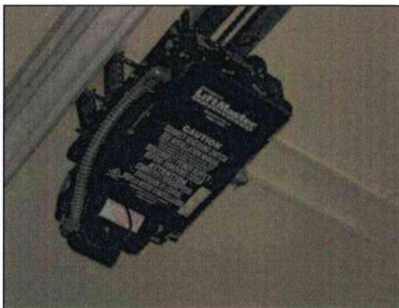
Photo 12 – Fire Station #4 The garage door is powered by an electronic Liftmaster opener. The unit appeared to function properly at the time of the inspection.
