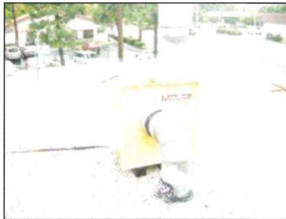
Photo 4 – Fire Station #4 The garage is ventilated by means of a vehicle exhaust system that is mounted on the roof. The system is similar to that present in Fire Station #5.
