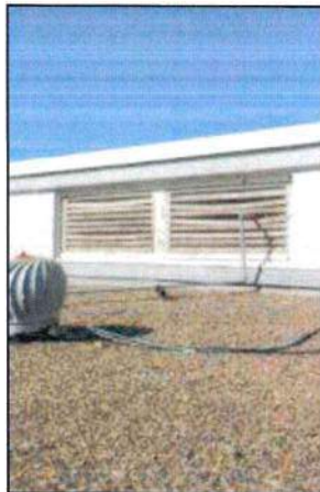
Photo 51 – Fire Station #1 Rooftop vent wood is buckled and rotted. The loose wiring should be run through conduit.
