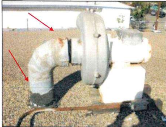
Photo 9 – Fire Station #1 The outside component of the vehicle exhaust system (GEF-6) is heavily corroded. The ducting requires sealant, and the flex joint requires a sheet metal shroud.
