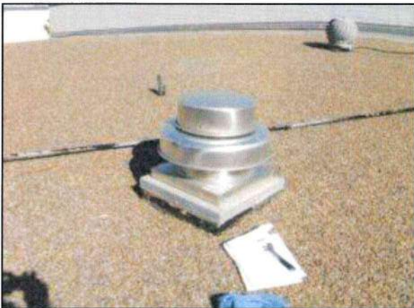
Photo 7 – Fire Station #1 A newly-installed exhaust fan (GEF-2) is present at the roof and is in good overall condition.
