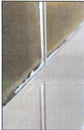
Photo 33 – Fire Station #1 Garage doors exhibit peeling and chipping of frame paint..
