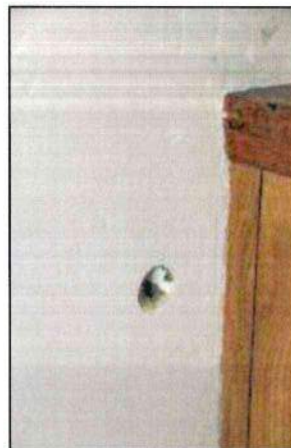
Photo 52 – Fire Station #1 Damage to the walls is present due to lack of door stoppers.
