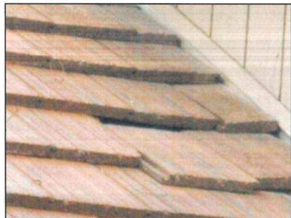
Photo 24 – Fire Station #4 Dislodged clay tiles were noted.
