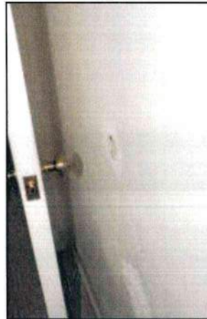
Photo 58 – Fire Station #1 The wall is damaged as a result of impacts from door handles.
