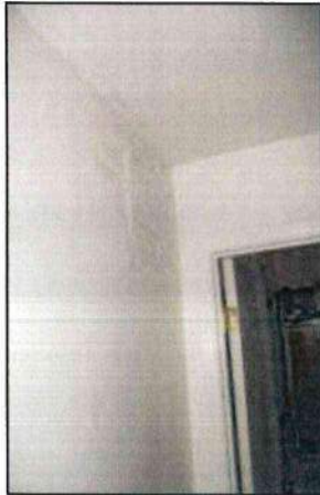
Photo 57 – Fire Station #1 Sections of wall patched with tape are present in the facility.
