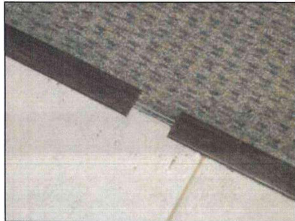
Photo 62 – Fire Station #4 The carpeting in the lounge area exhibits a damaged transition strip posing a potential trip hazard.
