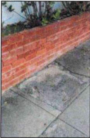
Photo 61 – Fire Station #1 Concrete sidewalk exhibits deterioration through scaling and spalling.
