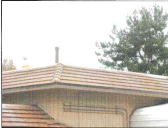
Photo 5 – Fire Station #4 The garage is ventilated by means of a vehicle exhaust system that is mounted on the roof. The system is similar to that present in Fire Station #5.
