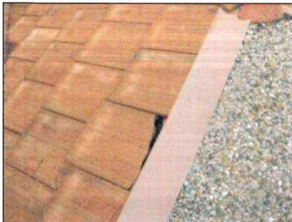
Photo 23 – Fire Station #4 Breaching of the tile roof was noted.
