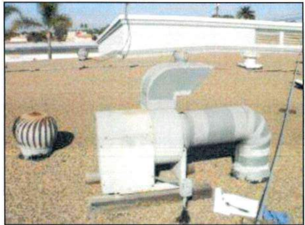
Photo 10 – Fire Station #1 A belt-driven, centrifugal type exhaust fan (GEF-3) requires sealant at the ducting.
