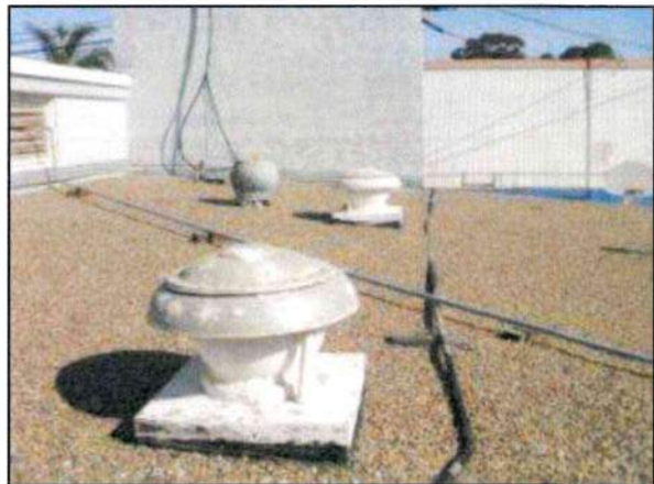
Photo 8 – Fire Station #1 Another exhaust fan (GEF-4) appears to be abandoned. Abandoned exhaust fans should be removed and permanently capped. Note GEF-5 in the background is also apparently abandoned in place.
