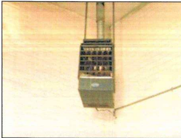
Photo 19 – Fire Station #1 A gas-powered space heater mounted on the wall of the garage is reported to be out of service, although it appears operational.
