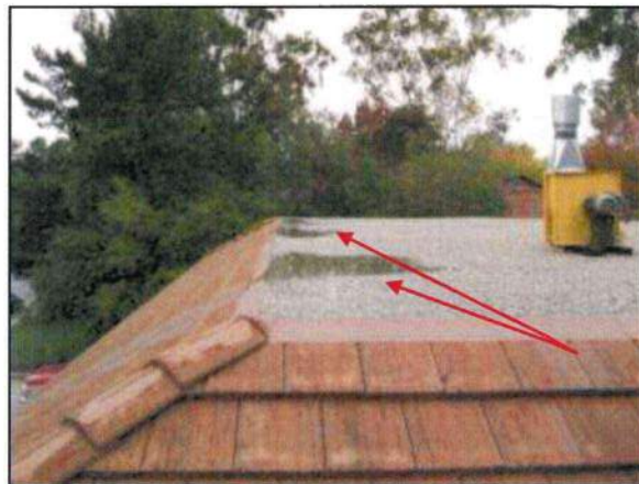
Photo 20 - Fire Station #4 Standing water was noted on the flat portion of the roof at the time of the inspection.
