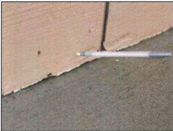
Photo 35 – Fire Station #4 Degraded T-111 siding is present near the base where it meets the concrete sidewalk slab.
