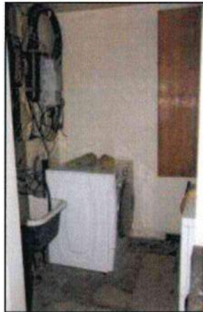
Photo 40 – Fire Station #1 The laundry room floor is completely deteriorated with missing sections and staining. The washer and dryer are not fitted with seismic straps.
