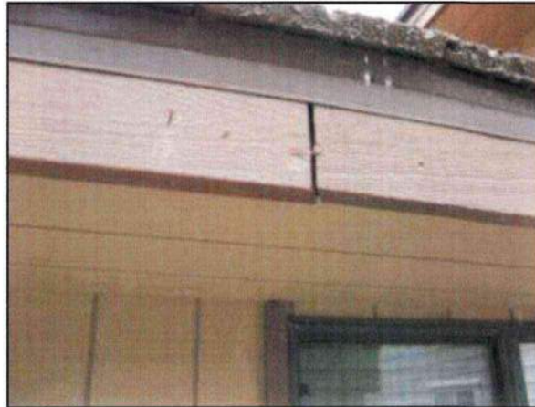
Photo 28 – Fire Station #4 The absence of a gutter system and separated fascia board was noted at the rear of the fire station.
