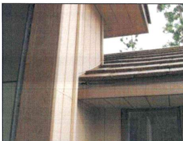
Photo 30 – Fire Station #4 The section of roof near the front entry exhibits poor flashing.
