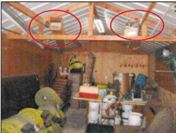
Photo 51 – Fire Station #4 No electrical sub panels are present in the storage shed. The electrical feed is from the main building. Note the fluorescent tube storage in the rafters.
