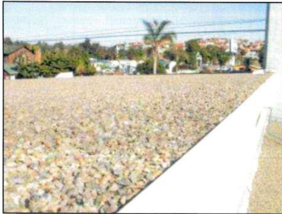
Photo 1 – Fire Station #1 The fire station exhibits a flat structure built up roof with gravel aggregate.
