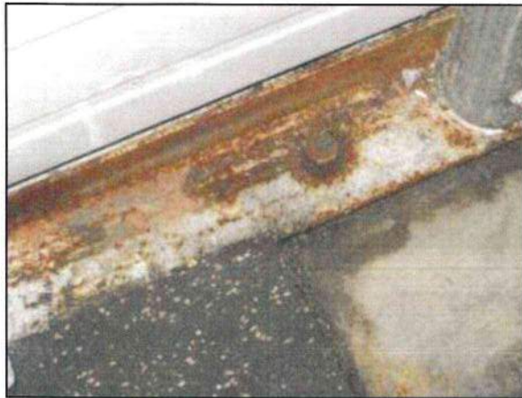
Photo 45 – Fire Station #4 Corrosion is present on the inside of the steel addition where it meets the slab as a result of poor sealing and lack of regular painting.
