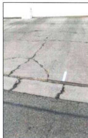
Photo 28 – Fire Station #1 The concrete at the garage is severely cracked and deteriorated. Loss of underlying support is also evident.
