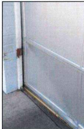
Photo 32 – Fire Station #1 Garage doors display evidence of impact damage.
