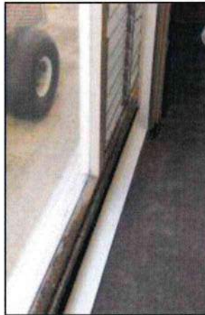
Photo 48 – Fire Station #1 Floor to ceiling windows exhibit deterioration of frames and water damage.
