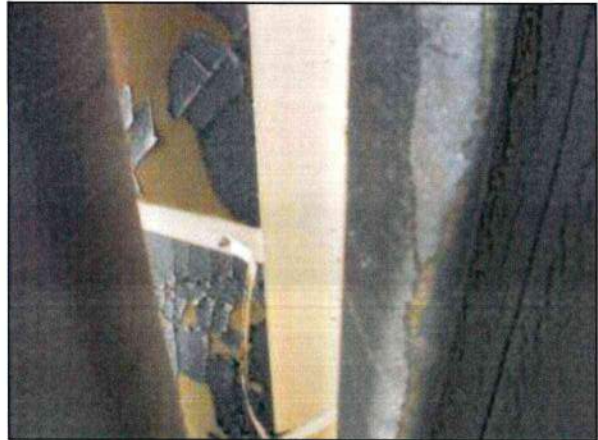
Photo 18 – Fire Station #1 Acoustical tiles located near the generator show signs of degradation.
