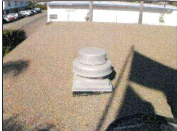
Photo 6 – Fire Station #1 An exhaust fan (GEF-1) is corroded, in poor condition, and may have been abandoned. Abandoned fans should be removed and their penetrations capped.
