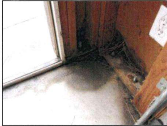
Photo 50 – Fire Station #4 Leaks are present inside of the storage shed at the entry door and at the wall where it meets the concrete slab.
