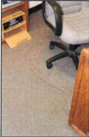
Photo 53 – Fire Station #1 Carpet generally lacks proper adhesion.
