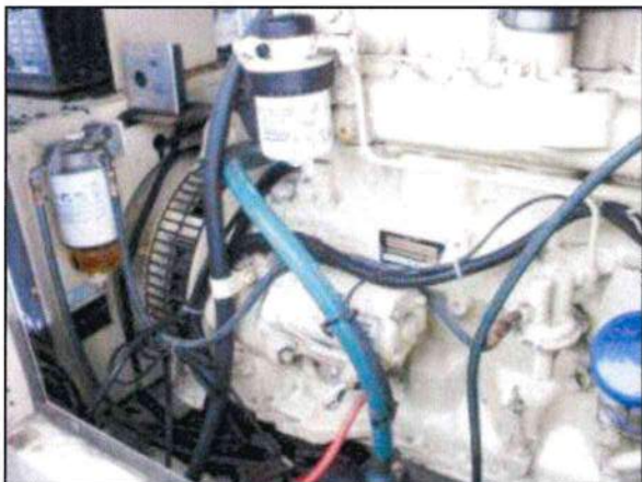
Photo 15 – Fire Station #1 The John Deere engine portion of the emergency generator system is equipped with a 120-gallon diesel fuel tank. It is in fair overall condition.
