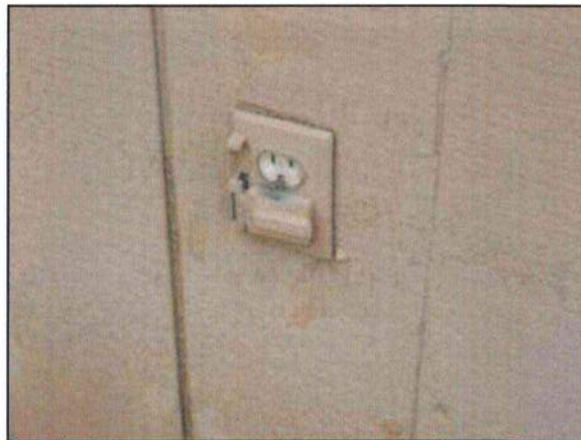
Photo 44 – Fire Station #4 The cover to an exterior outlet is missing and is not GFCI protected.
