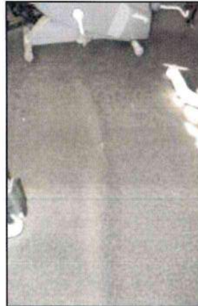
Photo 42 – Fire Station #1 The rolled rubber gym floor is not properly adhered to the base and lacks trim guards to prevent lifting and air pockets.
