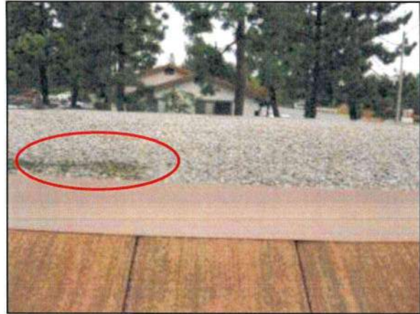
Photo 22 – Fire Station #4 Standing water was noted on the flat portion of the roof at the time of the inspection.
