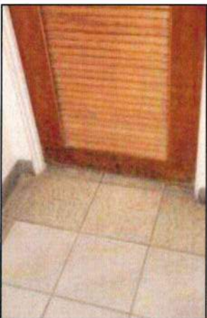
Photo 55 – Fire Station #1 The wood vented door to the restroom is stained and deteriorated. The floor is mismatched as a result of previous repairs of underground plumbing.
