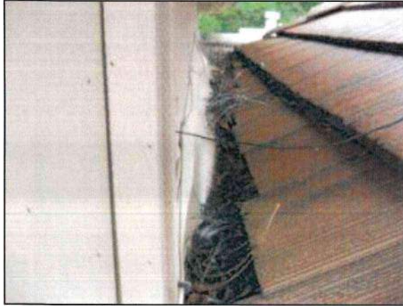
Photo 21 – Fire Station #4 The condition of the roof flashing is poor and the collection of tree litter will accelerate deterioration.
