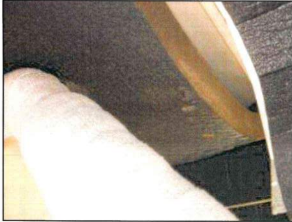
Photo 17 – Fire Station #1 Acoustical tiles located near the generator exhibit signs of degradation.
