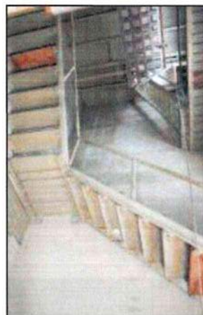
Photo 36 – Fire Station #1 Stairs in the hose tower have deteriorated and have been patched over time. Other sections require repairs.
