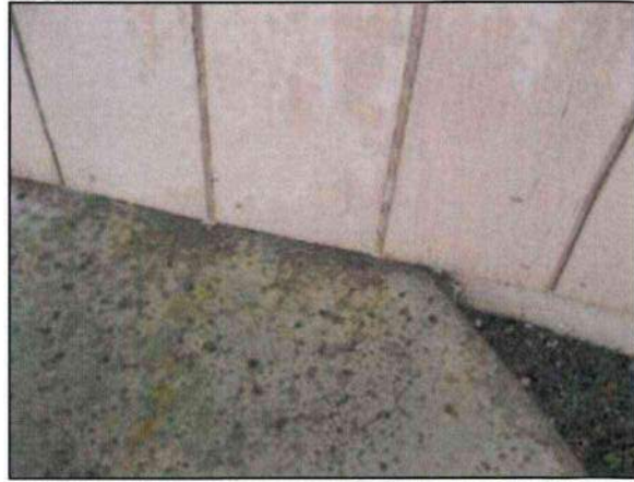
Photo 34 – Fire Station #4 The concrete sidewalk slab abuts the building sheathing.
