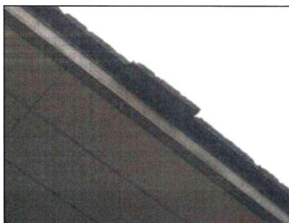
Photo 32 – Fire Station #4 Sections of roof with loose clay tiles were noted. These may present a hazard to those below.
