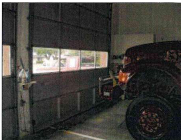
Photo 10 – Fire Station #4 The garage door is aged and exhibits repairs. Replacement of the door is recommended.
