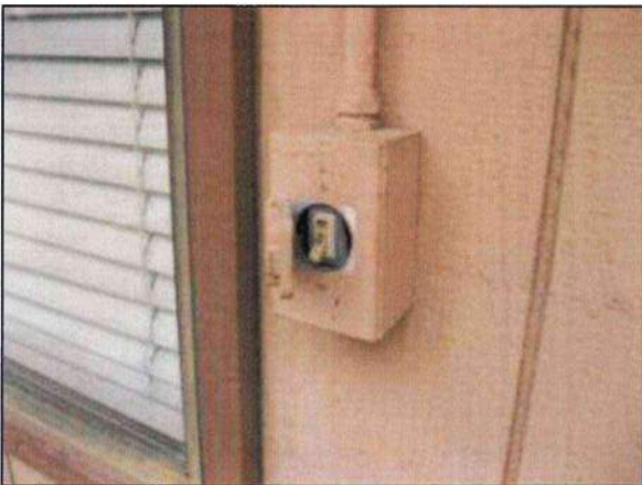
Photo 43 – Fire Station #4 The gasket to an exterior switch is missing.
