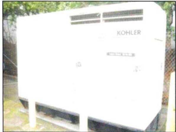
Photo 6 – Fire Station #4 The Kohler generator is located at the rear of the facility's site.
