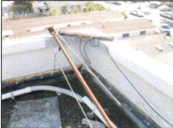
Photo 5 – Fire Station #1 A corner area of the roof needs the coping joints sealed, trash removed, and all penetrations sealed as a maintenance activity.
