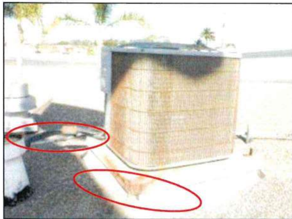
Photo 11 – Fire Station #1 The condenser portion of the split-system HVAC system located on the roof exhibits a rusted platform cap. The insulation for the refrigeration lines needs replacement.
