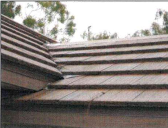
Photo 27 – Fire Station #4 “A general view of the new clay composition tile roof valley.
