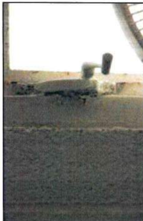
Photo 43 – Fire Station #1 Significant deterioration of window crank handles and frames is present.
