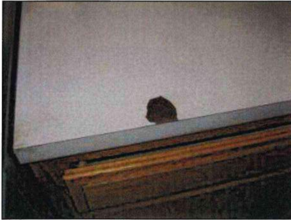
Photo 65- Fire Station #4 Damage to the Formica countertops in the kitchen is present.
