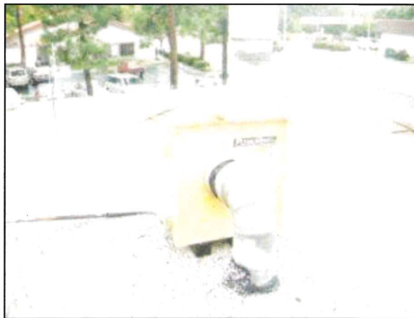
Photo 4 – Fire Station #4 The garage is ventilated by means of a vehicle exhaust system that is mounted on the roof. The system is similar to that present in Fire Station #5.
