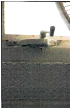
Photo 43 – Fire Station #1 Significant deterioration of window crank handles and frames is present.
