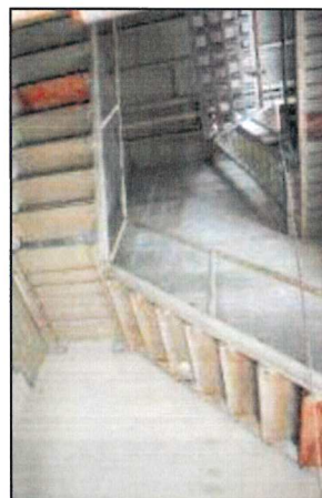
Photo 36 – Fire Station #1 Stairs in the hose tower have deteriorated and have been patched over time. Other sections require repairs.
