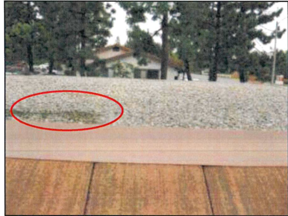
Photo 22 – Fire Station #4 Standing water was noted on the flat portion of the roof at the time of the inspection.
