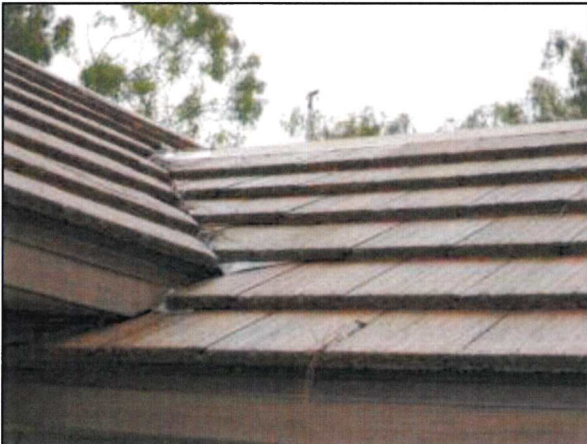
Photo 27 – Fire Station #4 “A general view of the new clay composition tile roof valley.
