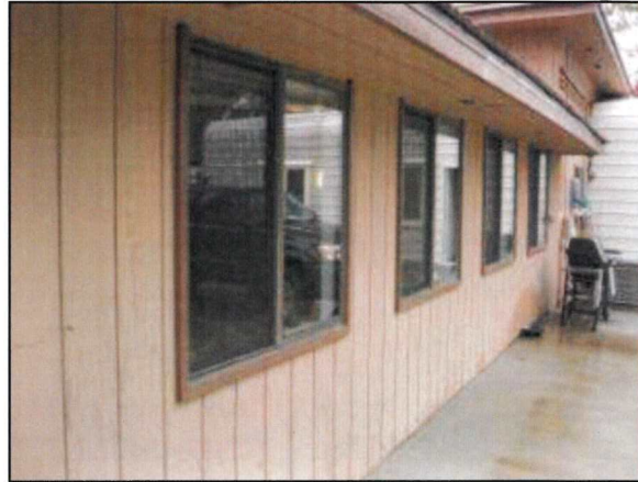
Photo 26– Fire Station #4 A general view of the rear of the fire station showing the aluminum window frames with insulated glass.
