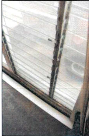
Photo 49 – Fire Station #1 Windows show deteriorated frames. The outdated louver windows allow air and moisture intrusion.
