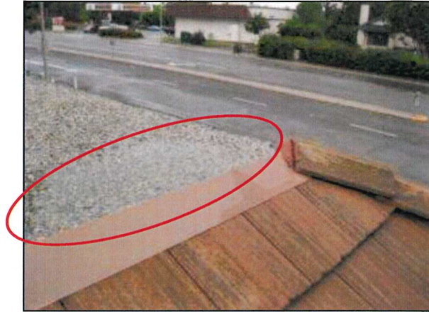
Photo 18 - Fire Station #4 Standing water was noted on the flat portion of the roof at the time of the inspection.
