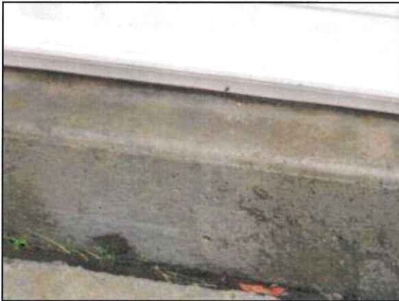
Photo 41 – Fire Station #4 The steel addition is not properly sealed to the concrete pad.
