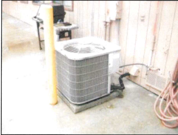
Photo 1 – Fire Station #4 The 3.5-ton condensing section is located at the rear of the facility and is paired with the furnace located in the bedroom closet.
