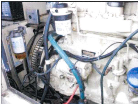
Photo 15 – Fire Station #1 The John Deere engine portion of the emergency generator system is equipped with a 120-gallon diesel fuel tank. It is in fair overall condition.
