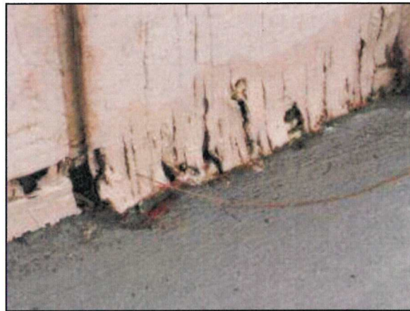
Photo 36 – Fire Station #4 Degraded T-111 siding is present near the base where it meets the concrete sidewalk slab.
