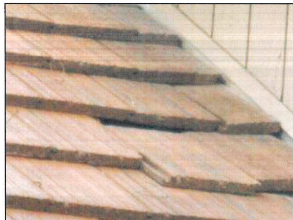
Photo 24 – Fire Station #4 Dislodged clay tiles were noted.
