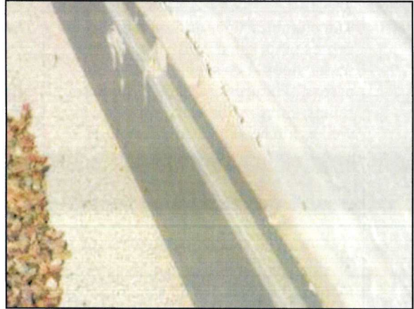
Photo 2 – Fire Station #1 Caulk repairs are needed at the termination flashing on the roof.
