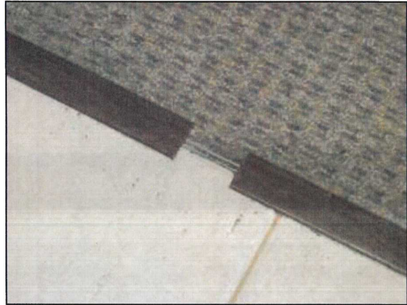
Photo 62 – Fire Station #4 The carpeting in the lounge area exhibits a damaged transition strip posing a potential trip hazard.
