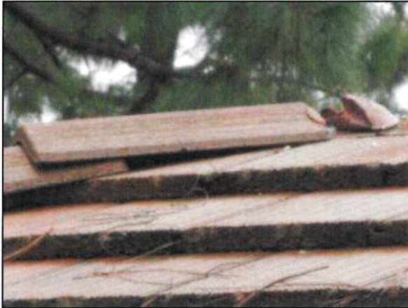
Photo 25– Fire Station #4 Unsecured roof tiles create points of entry for water as well as safety hazards below.
