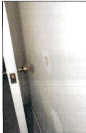
Photo 58 – Fire Station #1 The wall is damaged as a result of impacts from door handles.
