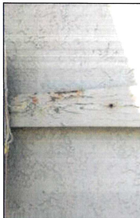
Photo 35 – Fire Station #1 Exterior wood trim exhibits cavitations, heavy rot and peeling of paint, and possible termite damage.
