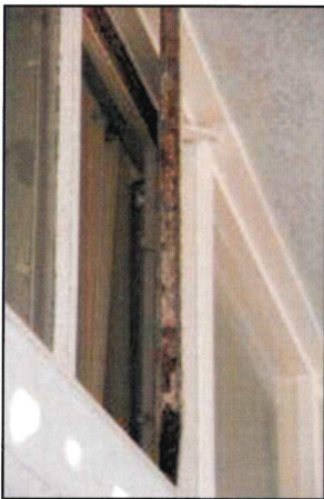
Photo 63 – Fire Station #1 Windows are significantly deteriorated with corrosion and peeling paint.
