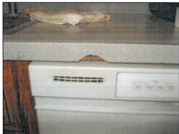
Photo 64 – Fire Station #4 Damage to the Formica countertops is present in the kitchen.
