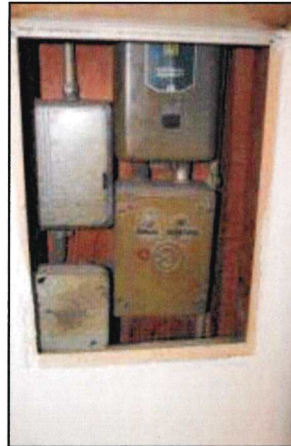
Photo 54 – Fire Station #1 A view of an electrical box within a wall.
