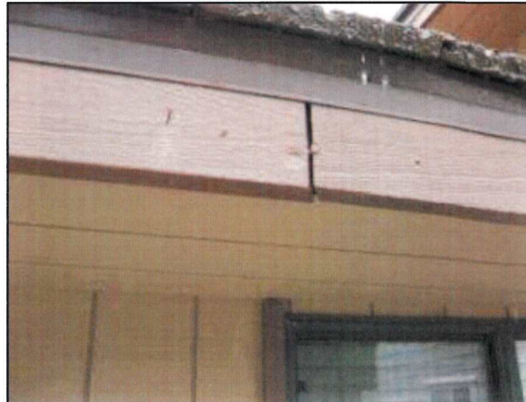
Photo 28 – Fire Station #4 The absence of a gutter system and separated fascia board was noted at the rear of the fire station.
