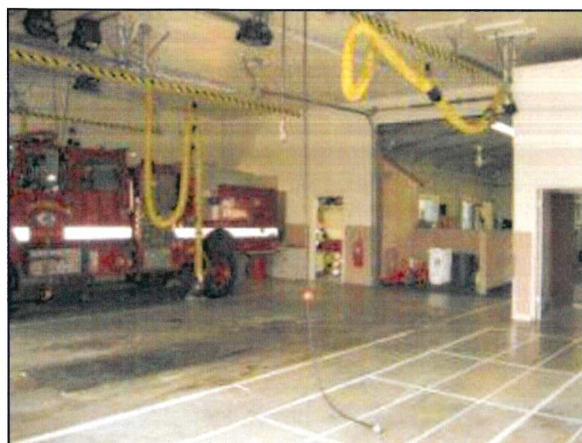
Photo 55 – Fire Station #4 A general view of the garage with the vehicle exhaust drops.
