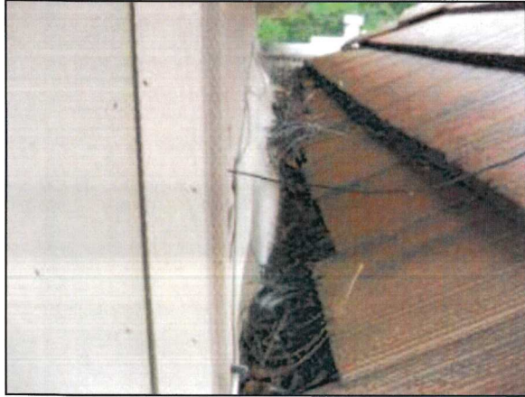
Photo 21 – Fire Station #4 The condition of the roof flashing is poor and the collection of tree litter will accelerate deterioration.
