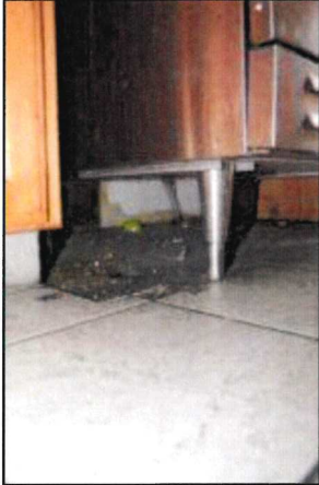
Photo 45 – Fire Station #1 Flooring around the kitchen range is missing and debris has accumulated.
