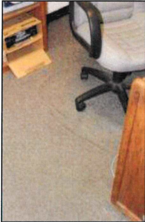
Photo 53 – Fire Station #1 Carpet generally lacks proper adhesion.
