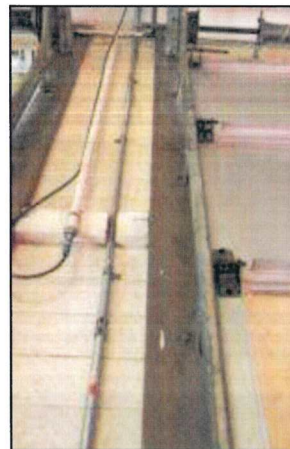
Photo 60 – Fire Station #1 Overhead door frames are deteriorated and have split as a result of age.
