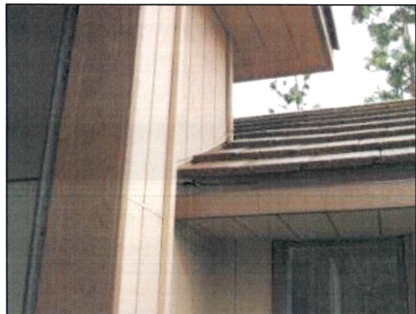
Photo 30 – Fire Station #4 The section of roof near the front entry exhibits poor flashing.
