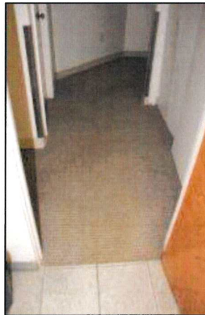
Photo 56 – Fire Station #1 Carpet in the living area hallway is worn and stained.
