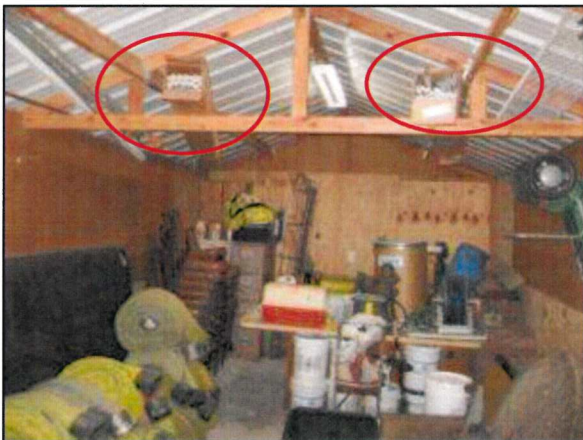
Photo 51 – Fire Station #4 No electrical sub panels are present in the storage shed. The electrical feed is from the main building. Note the fluorescent tube storage in the rafters.
