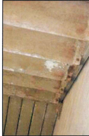
Photo 38 – Fire Station #1 Paint at the stairway shows severe peeling and flaking. Stair brackets are corroded.
