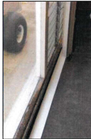
Photo 48 – Fire Station #1 Floor to ceiling windows exhibit deterioration of frames and water damage.
