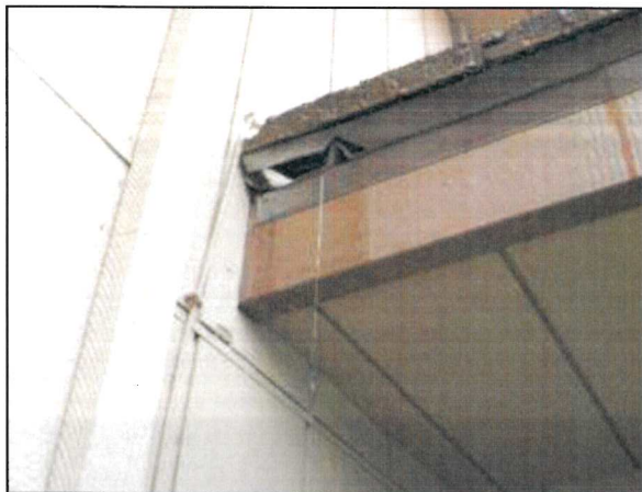
Photo 31 – Fire Station #4 The section of roof near the front entry exhibits poor flashing.
