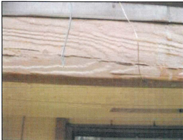
Photo 29 – Fire Station #4 Peeling paint and loose hanging wires were noted at the rear of the fire station.
