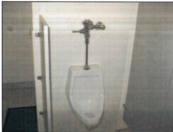
Photo 71– Fire Station #4 The urinal in the main restroom.
