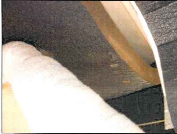
Photo 17 – Fire Station #1 Acoustical tiles located near the generator exhibit signs of degradation.
