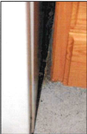
Photo 47 – Fire Station #1 Heavy debris has accumulated beside the refrigerator. The debris may attract pests.
