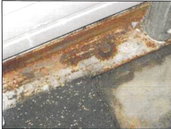
Photo 45 – Fire Station #4 Corrosion is present on the inside of the steel addition where it meets the slab as a result of poor sealing and lack of regular painting.
