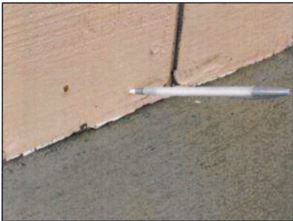
Photo 35 – Fire Station #4 Degraded T-111 siding is present near the base where it meets the concrete sidewalk slab.
