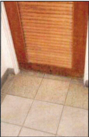
Photo 55 – Fire Station #1 The wood vented door to the restroom is stained and deteriorated. The floor is mismatched as a result of previous repairs of underground plumbing.
