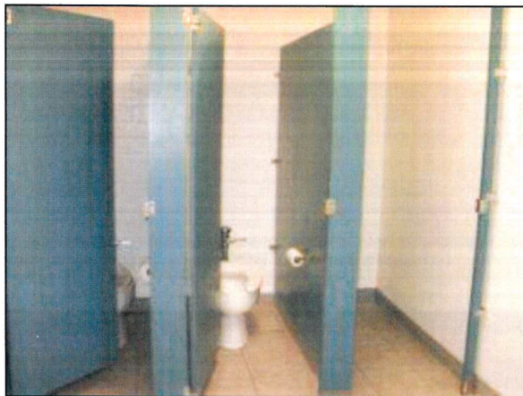
Photo 27 – Fire Station #1 A general view of the commodes in the locker room and general conditions.
