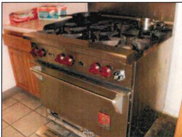
Photo 21 – Fire Station #1 The commercial-grade gas range and oven unit requires a thorough cleaning. The ceramic tile underneath requires repair in order to address sanitation.
