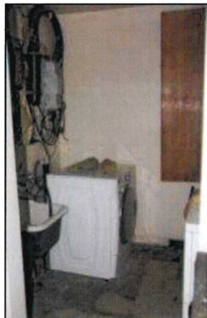
Photo 40 – Fire Station #1 The laundry room floor is completely deteriorated with missing sections and staining. The washer and dryer are not fitted with seismic straps.
