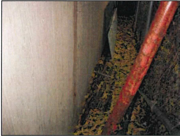
Photo 49– Fire Station #4 The back side of the storage shed is beginning to rot due to the presence of wet debris.
