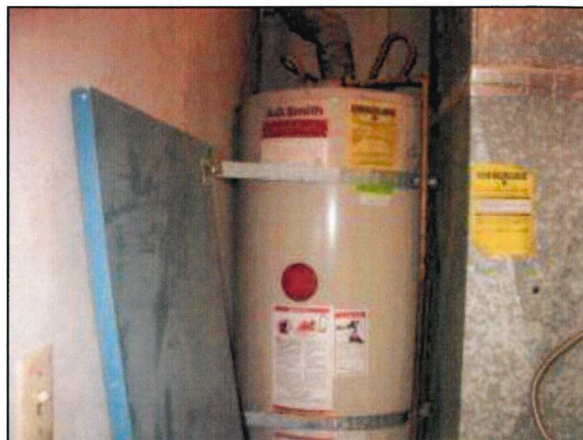
Photo 14 – Fire Station #1 The gas-fired water heater is located in the closet in the rest room.
