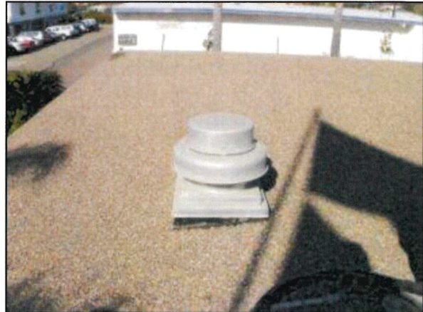
Photo 6 – Fire Station #1 An exhaust fan (GEF-1) is corroded, in poor condition, and may have been abandoned. Abandoned fans should be removed and their penetrations capped.
