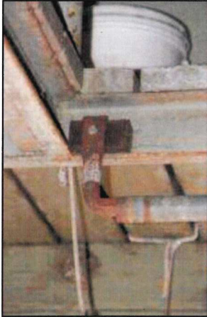
Photo 37 – Fire Station #1 Steel structural members of the stairways show significant rust.
