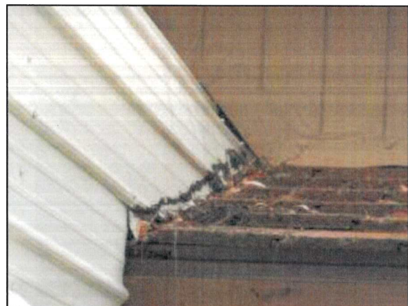
Photo 40 – Fire Station #4 A general view of the exterior where the steel addition attaches to the main building showing the improper flashing.
