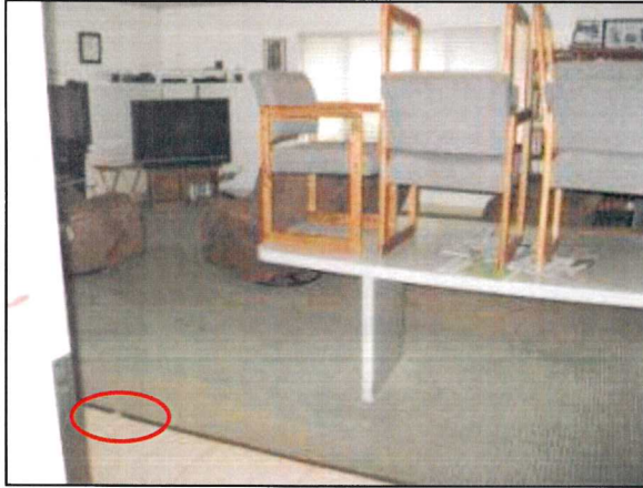
Photo 61 – Fire Station #4 A general view of the lounge area with a damaged carpet transition strip.
