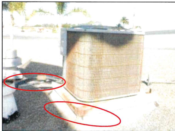
Photo 11 – Fire Station #1 The condenser portion of the split-system HVAC system located on the roof exhibits a rusted platform cap. The insulation for the refrigeration lines needs replacement.
