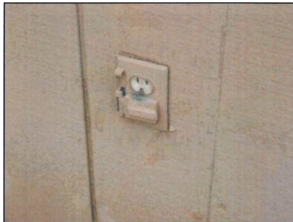
Photo 44 – Fire Station #4 The cover to an exterior outlet is missing and is not GFCI protected.
