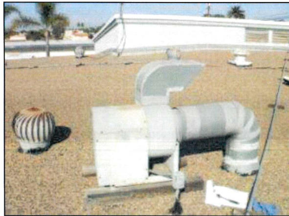
Photo 10 – Fire Station #1 A belt-driven, centrifugal type exhaust fan (GEF-3) requires sealant at the ducting.
