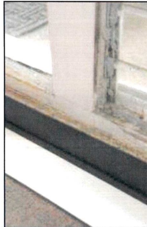
Photo 50 – Fire Station #1 Windows show deteriorated frames. The outdated louver windows allow air and moisture intrusion.
