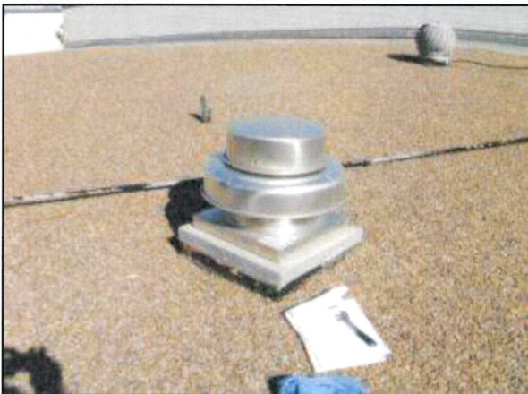
Photo 7 – Fire Station #1 A newly-installed exhaust fan (GEF-2) is present at the roof and is in good overall condition.
