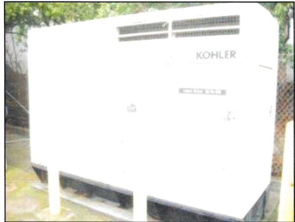
Photo 6 – Fire Station #4 The Kohler generator is located at the rear of the facility's site.
