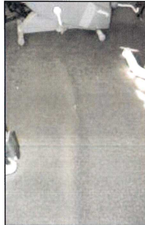
Photo 42 – Fire Station #1 The rolled rubber gym floor is not properly adhered to the base and lacks trim guards to prevent lifting and air pockets.
