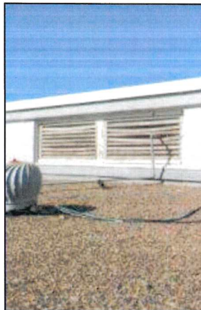
Photo 51 – Fire Station #1 Rooftop vent wood is buckled and rotted. The loose wiring should be run through conduit.
