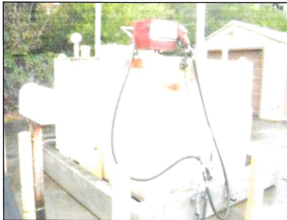
Photo 7 – Fire Station #4 A 1000-gallon fuel farm and dispensing system is present at the rear of the Station's site. The tank is above-ground and curbed.
