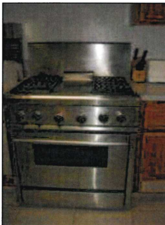
Photo 9 – Fire Station #4 A commercial kitchen range is located in the kitchen area. The unit was in good condition at the time of the inspection.
