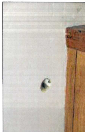
Photo 52 – Fire Station #1 Damage to the walls is present due to lack of door stoppers.
