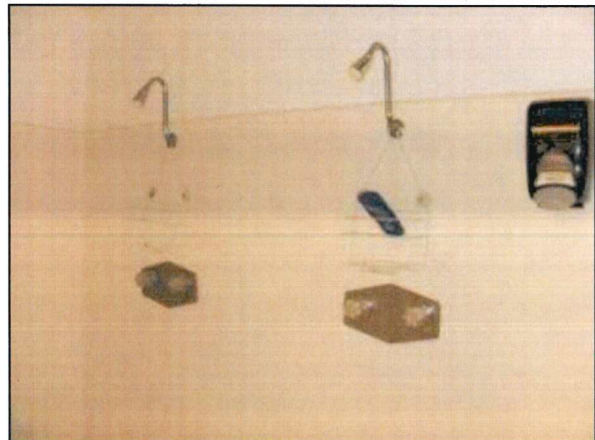
Photo 26 – Fire Station #1 A general view of the shower station in the locker room and general conditions.
