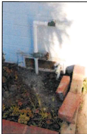
Photo 62 – Fire Station #1 Planters show some deterioration and loose bricks.
