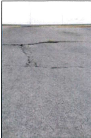
Photo 29 – Fire Station #1 The concrete at the garage is severely cracked and deteriorated. Loss of underlying support is also evident as a result of possible washout or settling.
