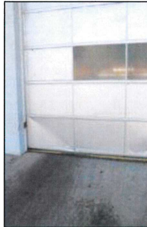
Photo 30 – Fire Station #1 Garage doors display evidence of impact damage.
