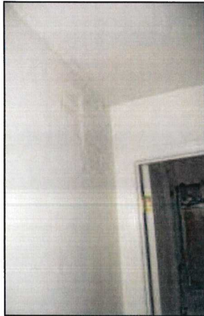
Photo 57 – Fire Station #1 Sections of wall patched with tape are present in the facility.
