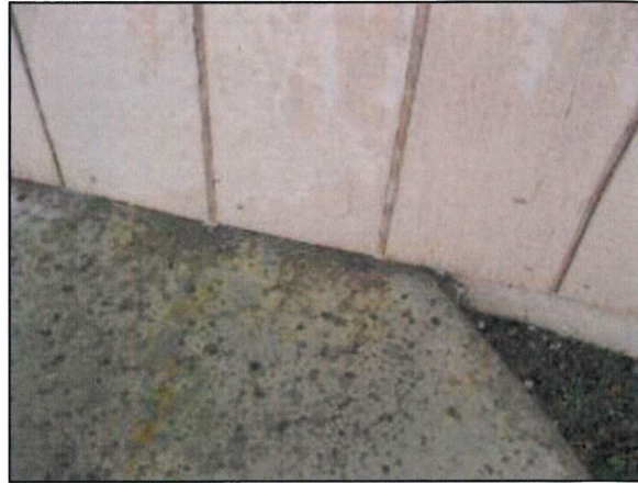
Photo 34 – Fire Station #4 The concrete sidewalk slab abuts the building sheathing.
