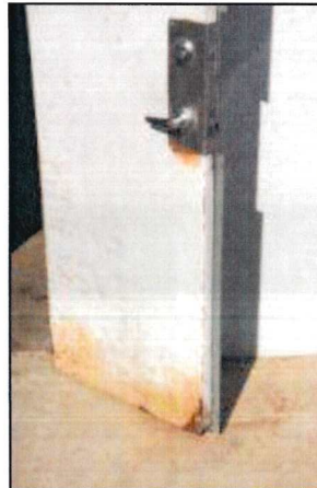
Photo 34 – Fire Station #1 The exterior door to the hose tower is significantly rusted.
