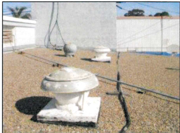
Photo 8 – Fire Station #1 Another exhaust fan (GEF-4) appears to be abandoned. Abandoned exhaust fans should be removed and permanently capped. Note GEF-5 in the background is also apparently abandoned in place.
