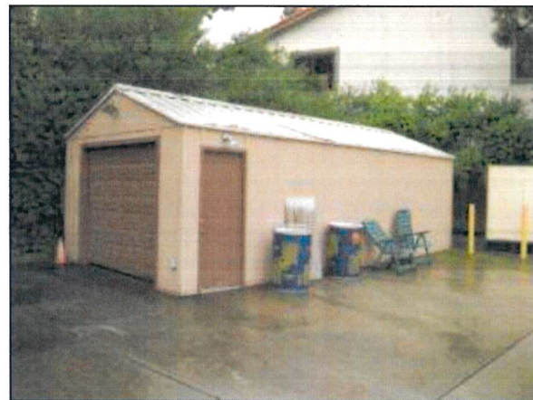
Photo 48 – Fire Station #4 The storage shed located at the rear of yard is sheathed in T-111 masonite and has a steel roof, steel entry door, and an aluminum roll-up door.
