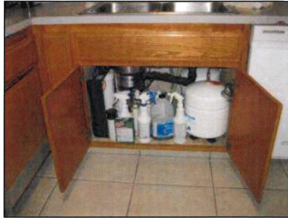
Photo 66 – Fire Station #4 The kitchen sink is equipped with a garbage disposal and reverse osmosis water filtration system.
