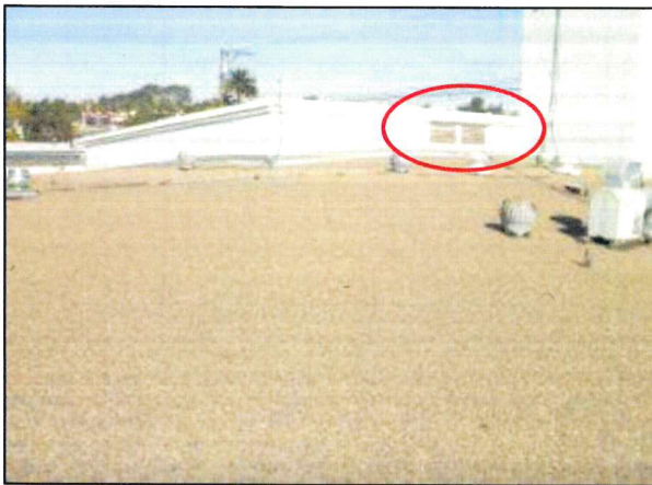
Photo 3 – Fire Station #1 Wood louvers present at the roof are deteriorating and need to be repainted.
