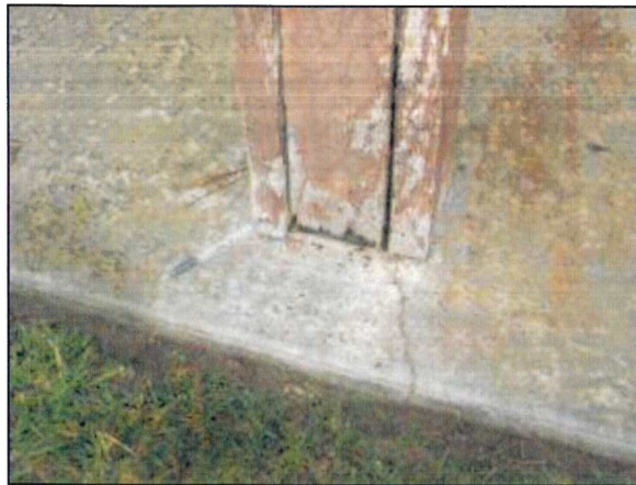
Photo 47 – Fire Station #4 A structural post located at the front porch is rotted at the base.
