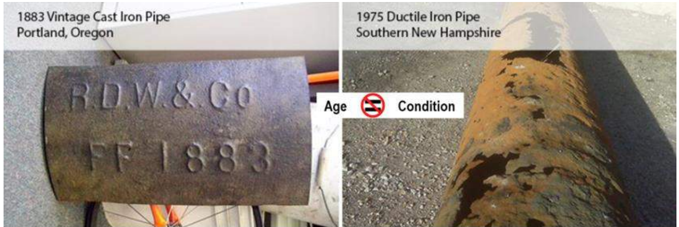
Figure 7-6. Age Alone is a Poor Indicator of Pipe Condition and Remaining Useful Life
